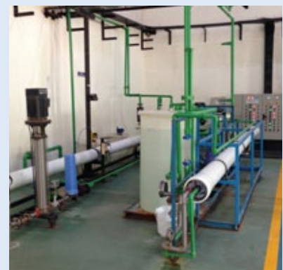
Secondary Reverse Osmosis plant
